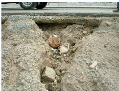
Undermining of road as a consequence of an untreated sodic and saline soil.
