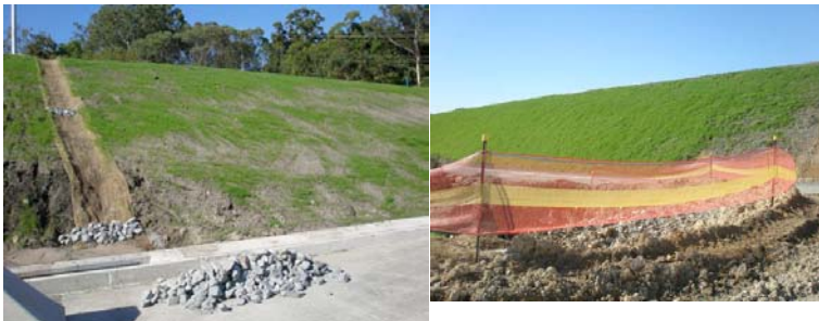
LH photo shows hydro-seeding with specified mix. RH photo shows hydro-seeding with modified mix as a result of a soil test to reflect actual soil requirements.
