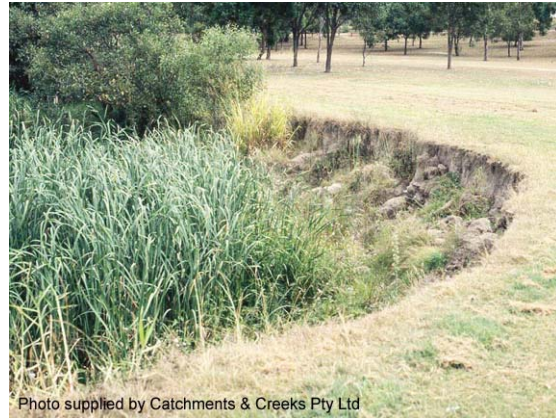
Photo 4 – Bank scour on channel bend
