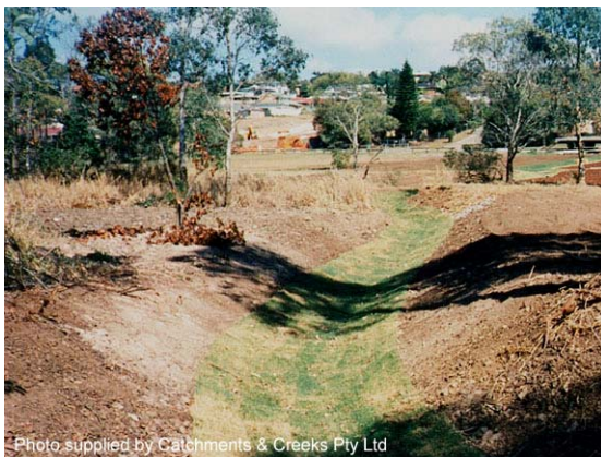
Photo 9 – Grass-lined, parabolic drain
