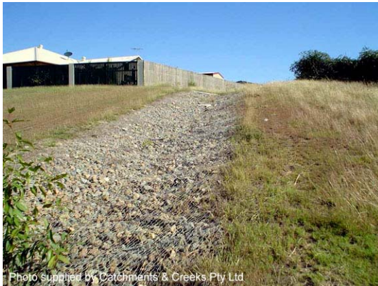
Photo 15 – Permanent rock mattress drainage chute
