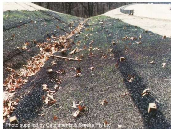
Photo 2 – Permanent, synthetic reinforced erosion control mat
